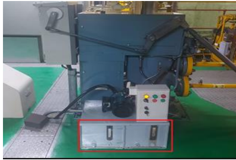
Gambar 10. Governor Sistem dan Leakage Oil Pump.
