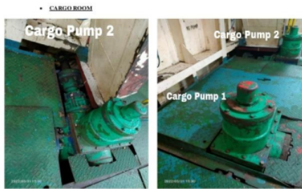
Gambar 2. Cargo Pump 1 dan Cargo Pump 2
